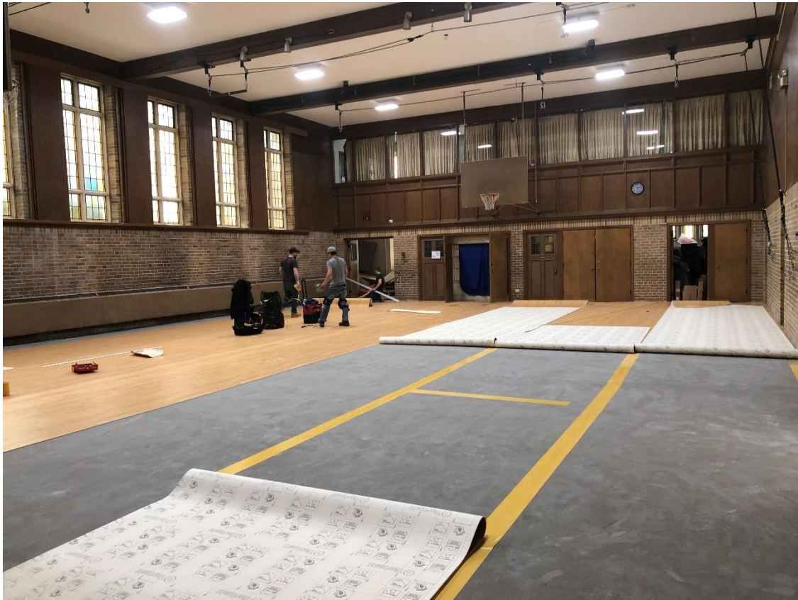
Here is the gymnasium with the new floor and new ceiling. Lighting and lines on the gym floor are presently being applied.
